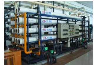
RO Process Water Treatment Plant
