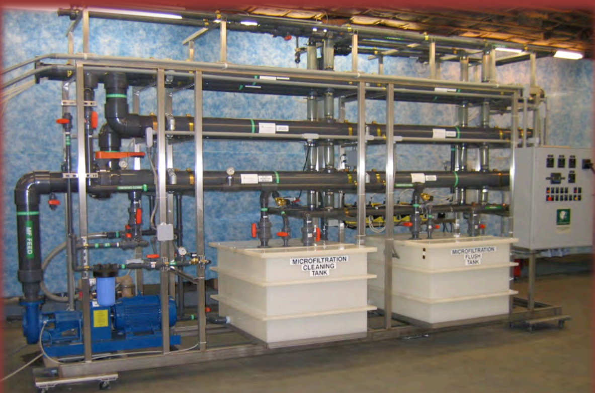
Figure 1 – Duraflow System Showing Tanks and Piping for Membrane Cleaning
